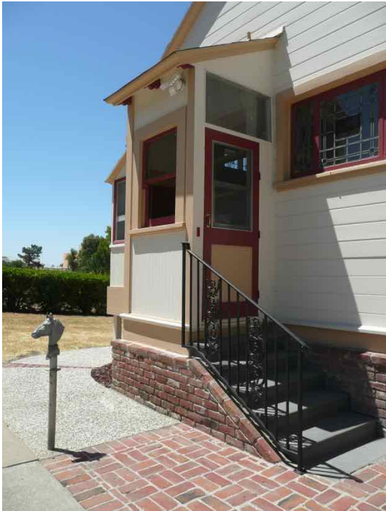
Early shed roof addition (rear entry portico) at east elevation of gabled addition, facing southwest.
