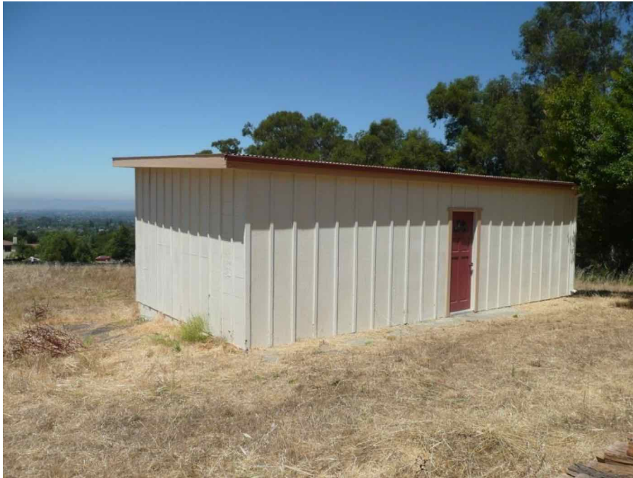
South and east elevations of the contemporary horse tack building, facing northwest.
