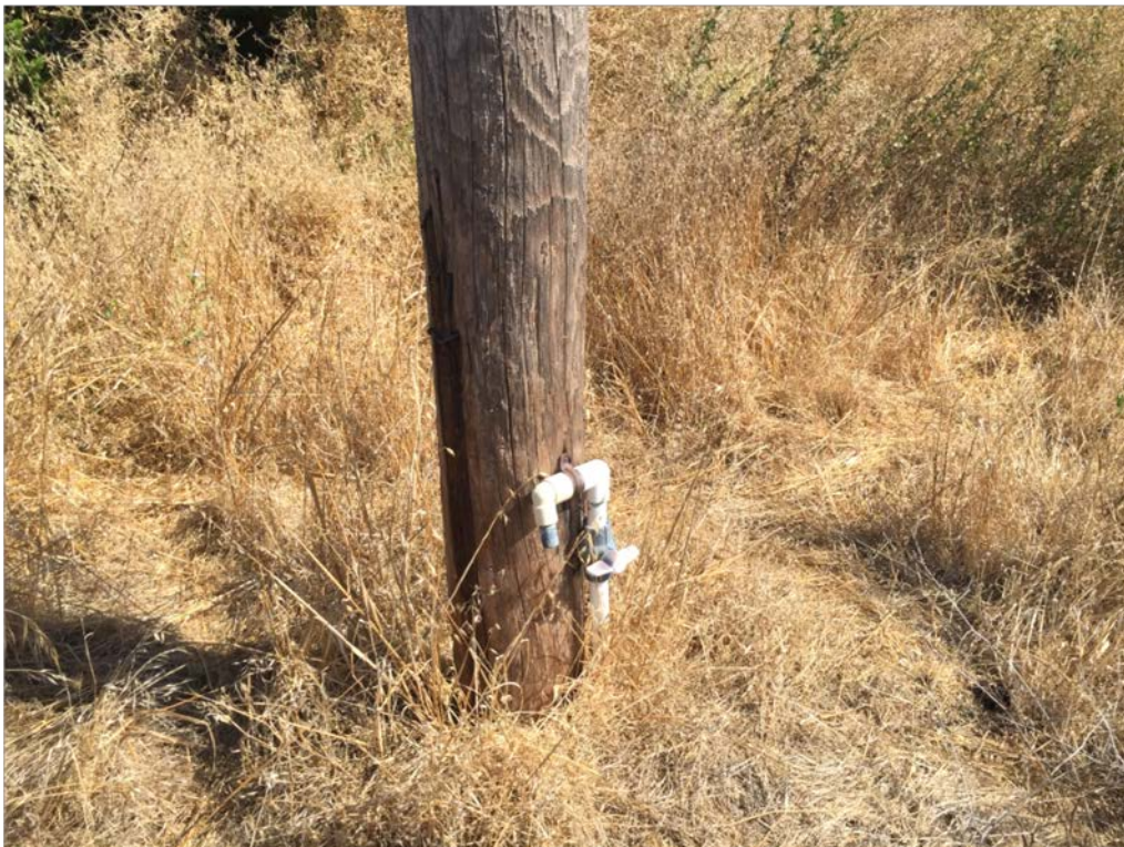
Photograph 9. Piping near water well. Piping is no longer connected to well.
