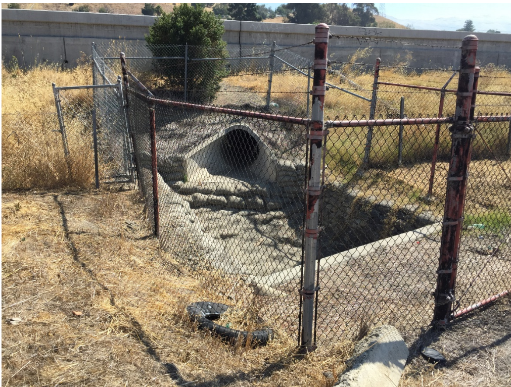
Photograph 11. Drainage catch basin observed along the eastern border of the Site adjacent to Highway 680.
