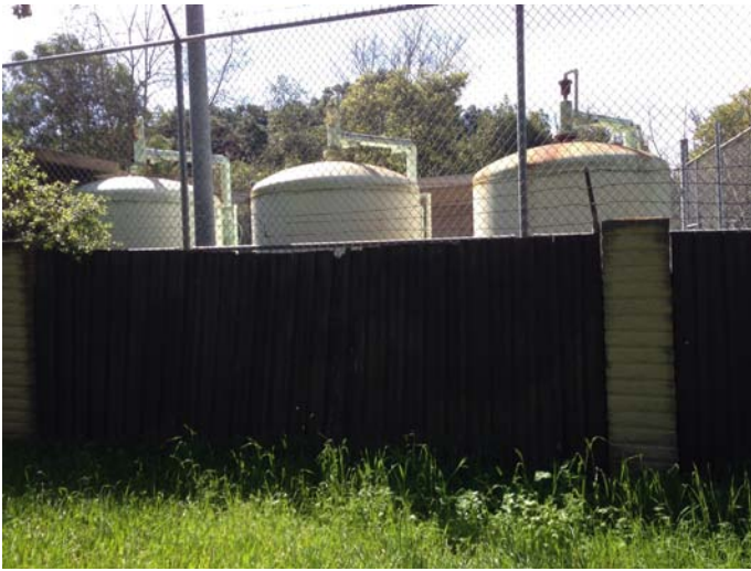
Closer look at ACWD well compound
