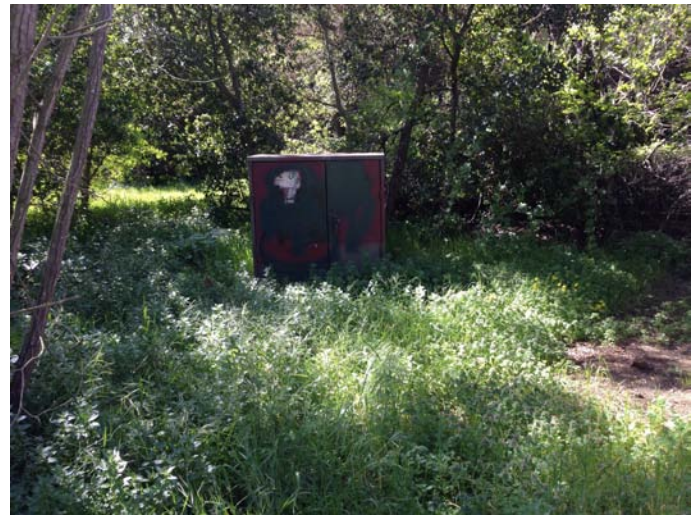
Transformer next to ACWD compound
