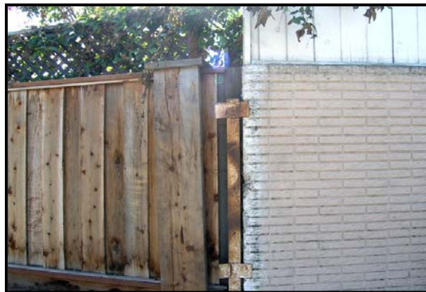
Figure 6: Incompatible Fence Materials
