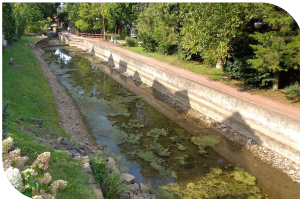
Storm water canals
