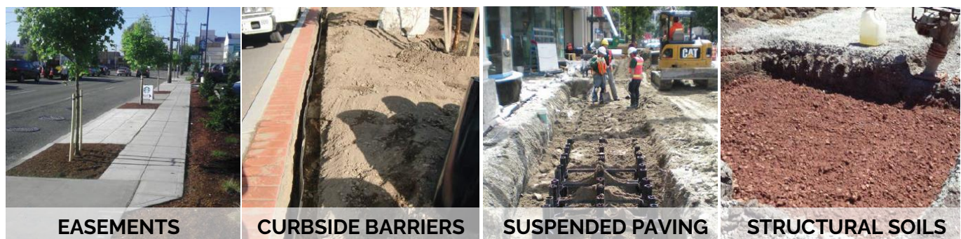
Image Description 24. Examples of the potential alternative solutions for tree and hardscape conflicts
