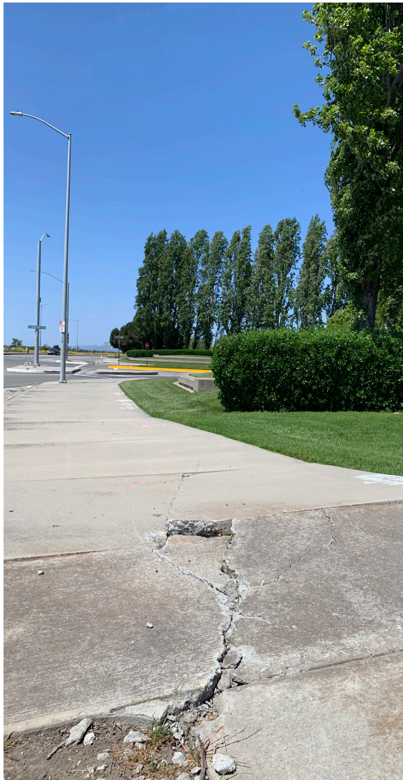
Damaged sidewalk on Paseo Padre Parkway near Dumbarton Circle
