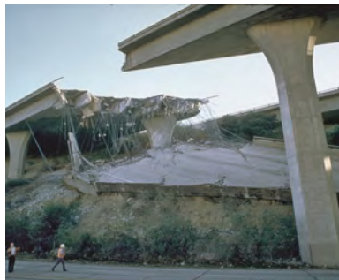
Earthquake damage to transportation infrastructure
