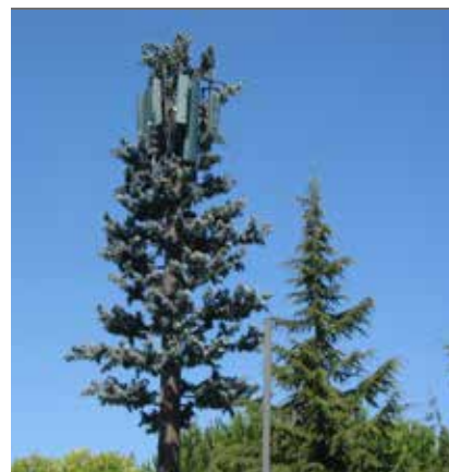
The above two faux trees have exposed antennas with no covers or needle socks and insufficient foliage and branches to hide equipment.
