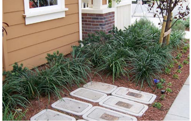
RECOMMENDED - Well-organized clustered utilities in a well-landscaped unobtrusive location.
