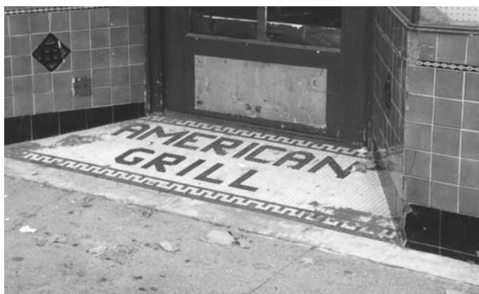
Figure 22 An example of a tile-clad bulkhead and recessed entry to a Niles restaurant
